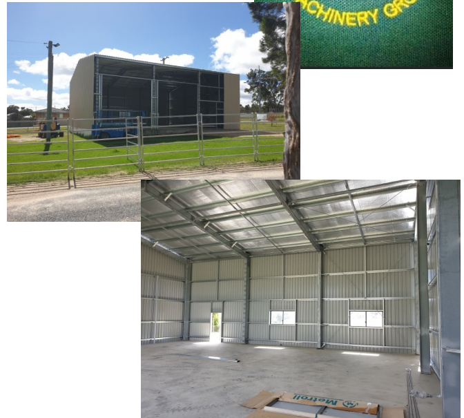
Above: Images of the new shed courtesy of the Stanthorpe Historical Vehicle and Machinery Group.
